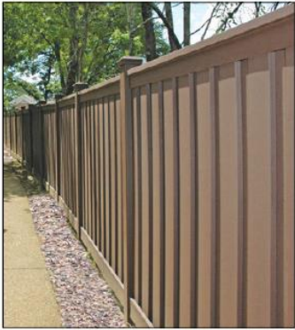
On this page are various views of the Burton Hills installation. (Rio Grande Fence photos)
